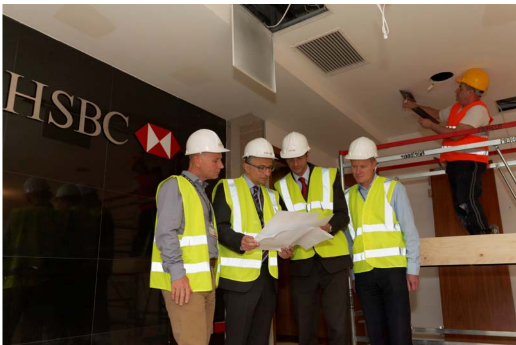
Nikolaos Fertakis - Chief Operating Officer HSBC Bank Malta (second from left) together with Dale Jephson, Ivan Borg and Michael J Cassar inspecting the works in progress at the new corporate banking centre in Qormi
