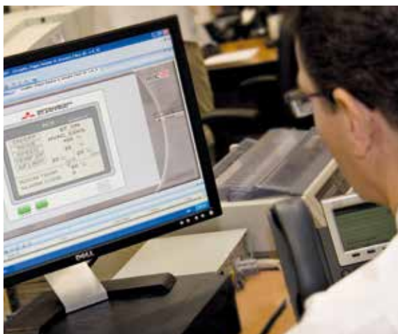
Victor Friggieri, HSBC's Manager for Energy and Sustainability and winner of the 2012 Worker of the Year Award, demonstrates HSBC Malta's Building Management System which significantly reduces energy consumption in HSBC Malta's buildings and branches.
